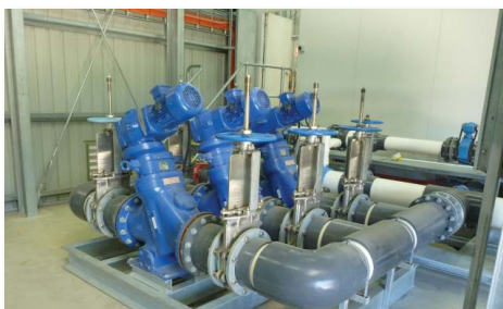
Control Shed - Inline Grinders
