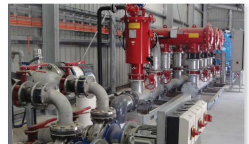
Control Shed - Tertiary Treatment
